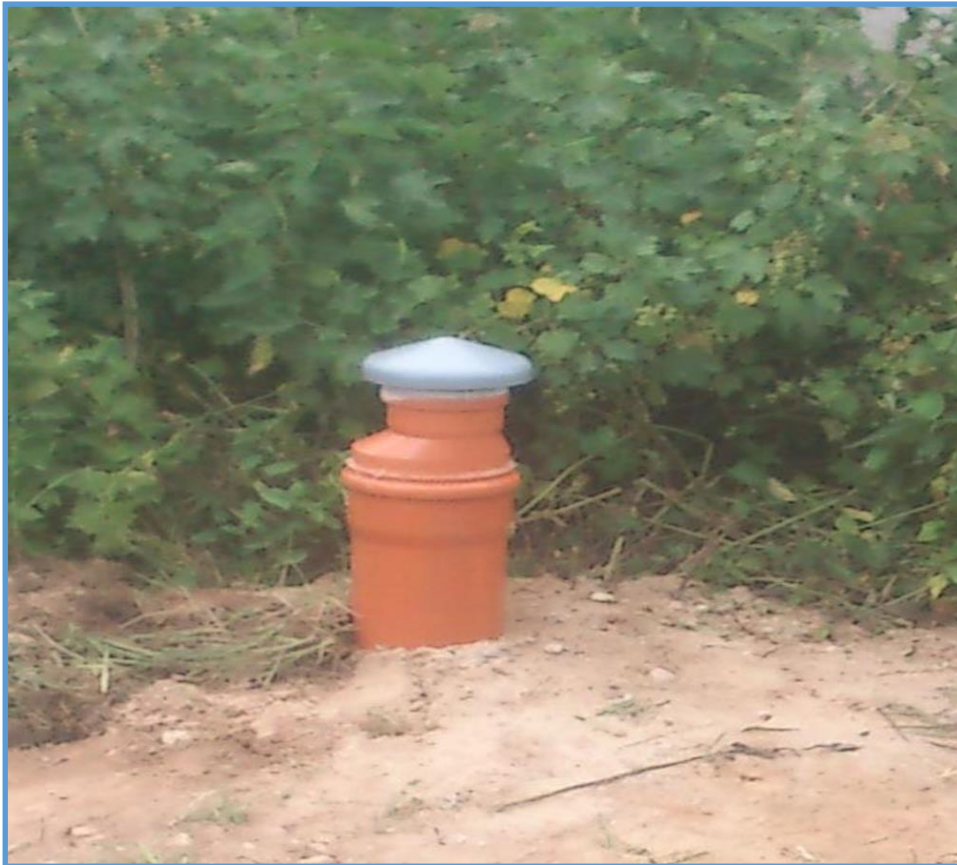
Common view of the site of a buried seismometer installation
